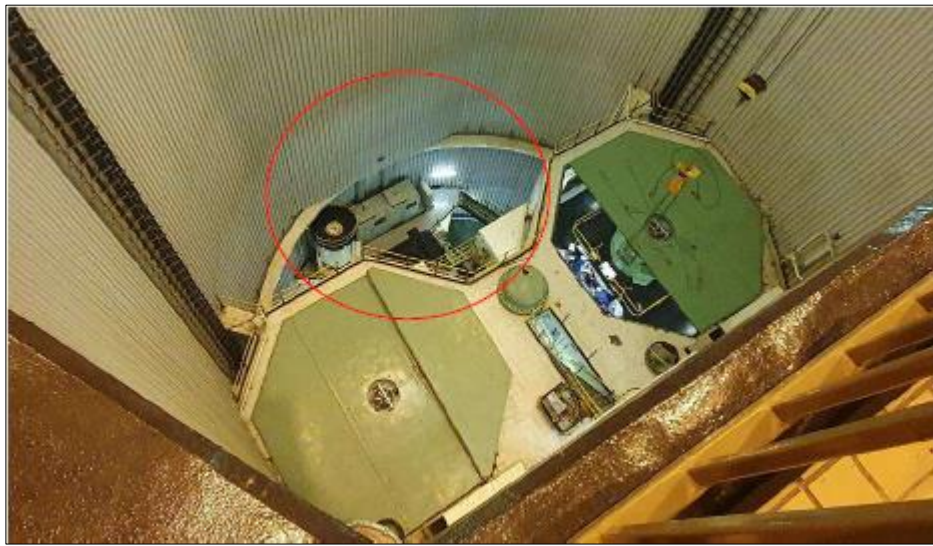
Figure 6 Location of the compressor within the turbine shaft as viewed from ground level.
