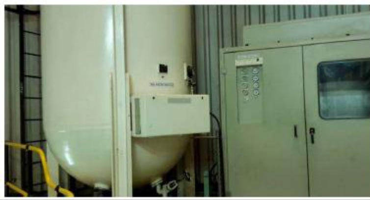
Figure 4 Compressor sound enclosure and air vessel.
