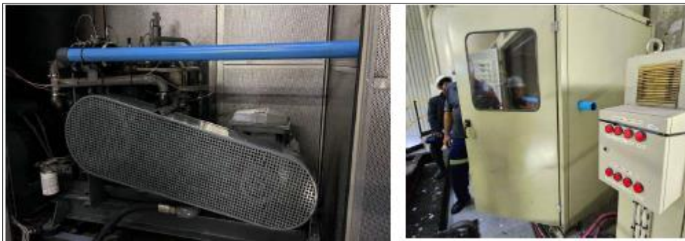
Figure 3 Image of LMF compressor in sound enclosure, including modification of air infeed to reduce air temp at inlet.
