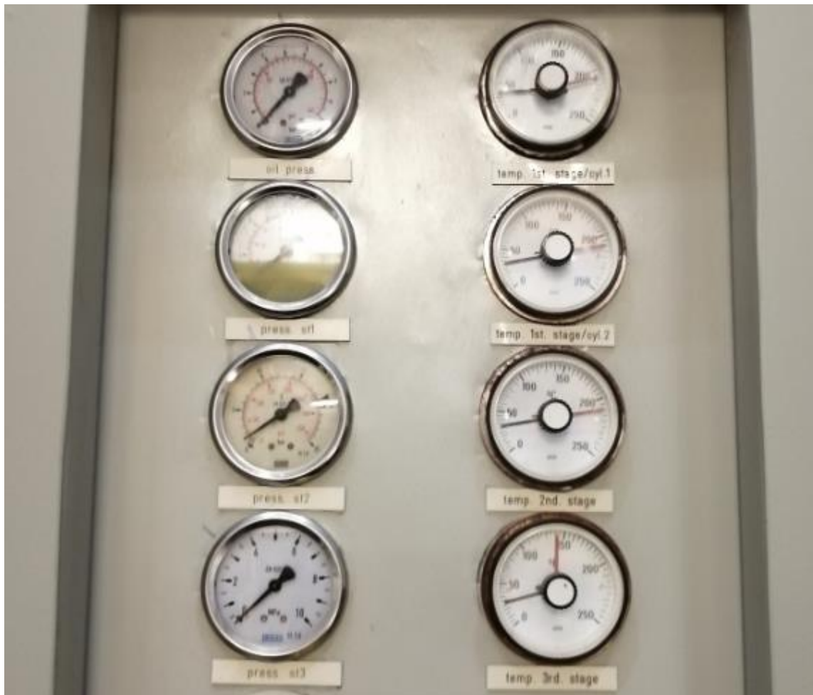
Figure 9 Performance monitoring on current compressor.
