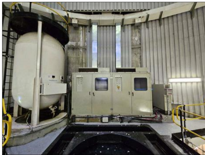
Figure 7 Positioning of the compressor as viewed from the turbine level.
